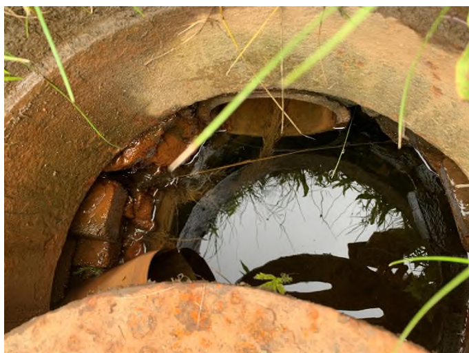
CB - 2 (Catch Basin)
