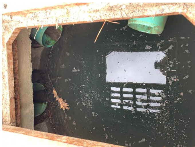
CB - 1 (Catch Basin)
