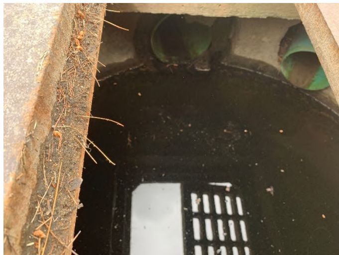
CB – 1 (Catch Basin)
