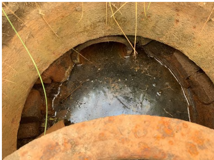
CB – 2 (Catch Basin)
