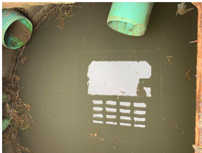
CB - 1 (Catch Basin)
