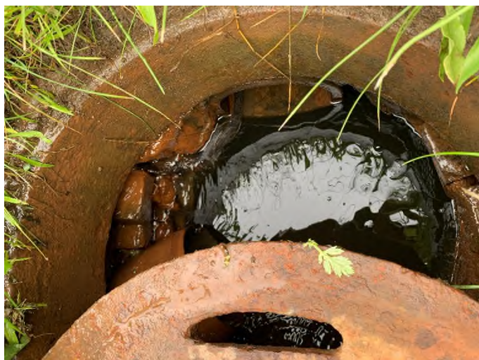
CB – 2 (Catch Basin)
