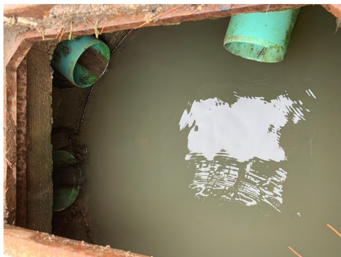
CB – 1 (Catch Basin)
