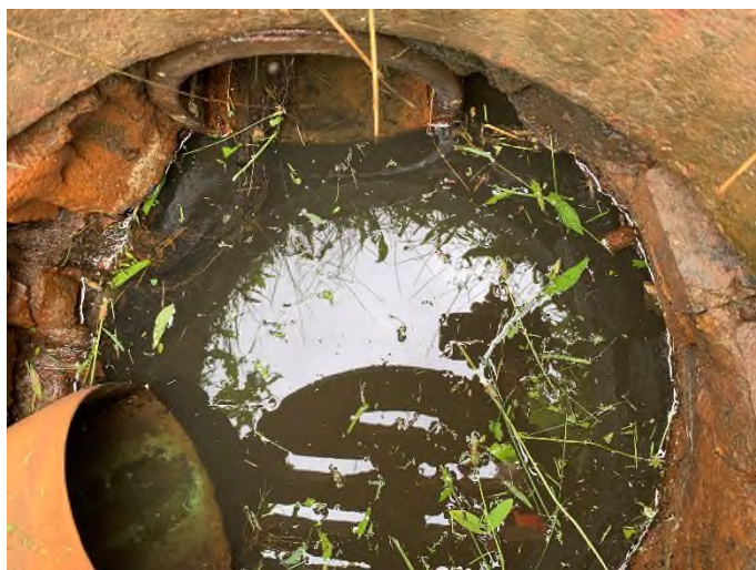
CB - 2 (Catch Basin)
