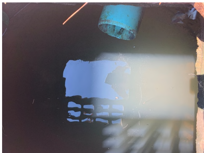
CB – 1 (Catch Basin)
