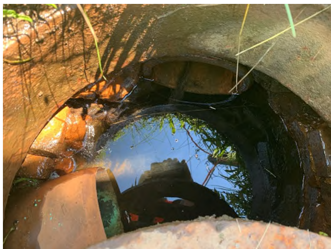
CB – 2 (Catch Basin)
